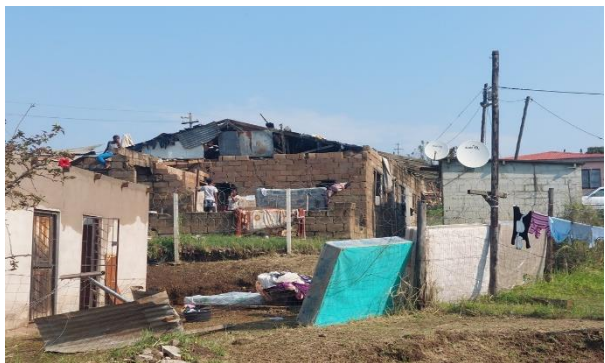
Roofs in some of the residential homes at Inanda Durban, were uprooted during a tornado that ripped through the townships
